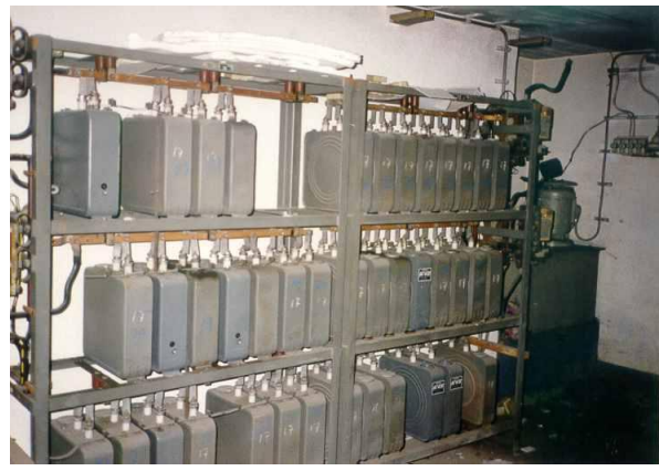
Closed systems, example capacitor battery
